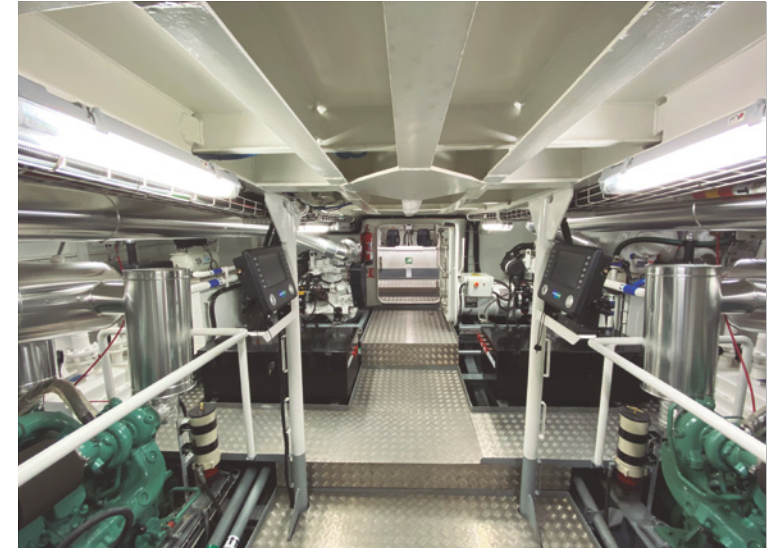
ENGINE ROOM. Ample work space for the crew.
