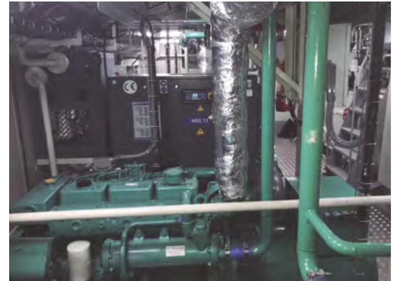
MACHINE ROOM. Ample work space for the crew.
